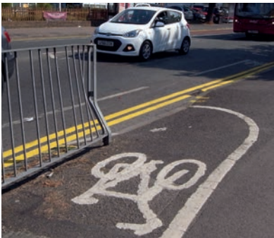
Cycle lanes are poorly marked and stop abruptly
