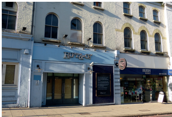
Loss of historic features at ground level
